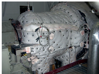
Fig. 16. Shell warming system providing faster steam turbine start times
